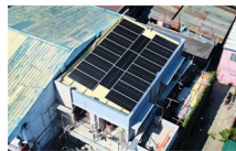
10kW Solar Grid-Tied System Sta. Maria, Bulacan
