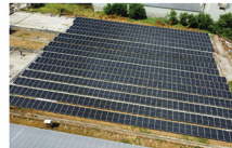
300kW Solar Grid-Tied System San Miguel, Bulacan
