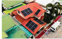
5kW Solar Grid-Tied System San Fernando, Pampanga
