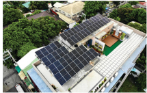
25.02kW Solar Grid-Tied System Malate, Manila
