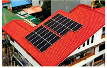
10kW Solar Grid-Tied System Sta. Ana, Manila
