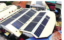
200kW Solar Grid-Tied System Caloocan City
