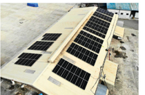
100kW Solar Grid-Tied System San Jose, Nueva Ecija
