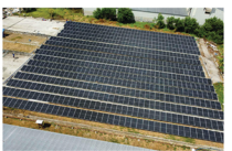
300kW Solar Grid-Tied System San Miguel, Bulacan
