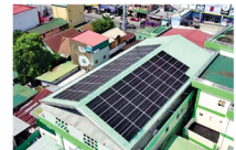
50kW Solar Grid-Tied System San Ildefonso, Bulacan
