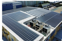
1.5MW Solar Grid-Tied System Muntinlupa City
