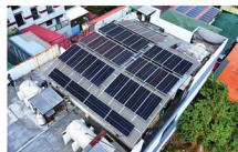
20kW Solar Grid-Tied System Quezon City
