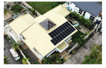
10kW Solar Grid-Tied System Angeles, Pampanga
