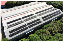
200kW Solar Grid-Tied System Bacnotan, La Union
