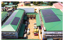
180kW Solar Grid-Tied System Quezon City
