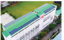
99kW Solar Grid-Tied System Caloocan City
