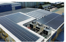
1.5MW Solar Grid-Tied System Muntinlupa City
